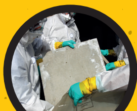
ASBESTOS MILLBOARD AND PAPERS
